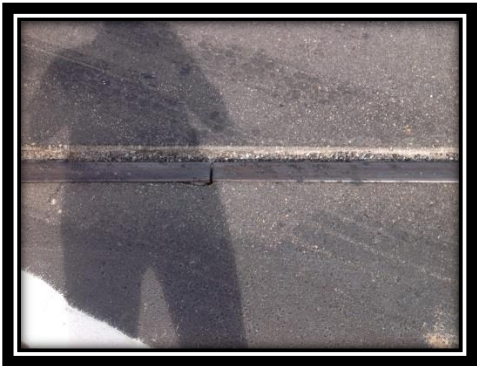
Railroad Crossing Hazard (On Fields)
