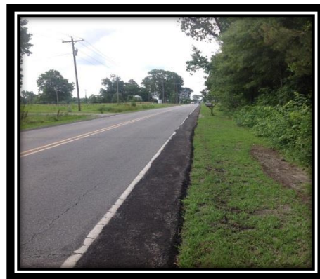
Narrow Shoulder Hazard (Moye-Turnage)
